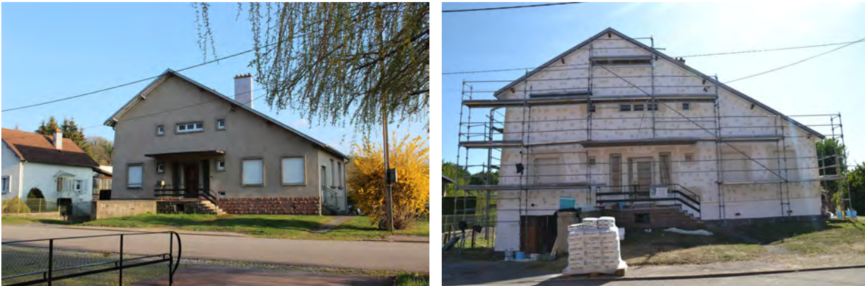
Figure 8a and 8b. Saulcy-sur-Meurthe. The presbytery before (on the left) and after (on the right) the external isolation with polystyrene panels and coating, 2019-2021 (photograph by the authors)
